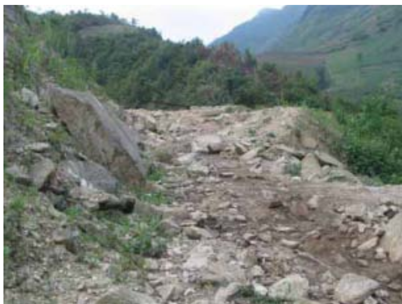
View of a badly damaged inaccessible road leading to school. Girls are made particularly vulnerable by physical challenges in getting to school. Photo taken at Thai Giang Pho commune, Bac Ha district, Lao Cai province
