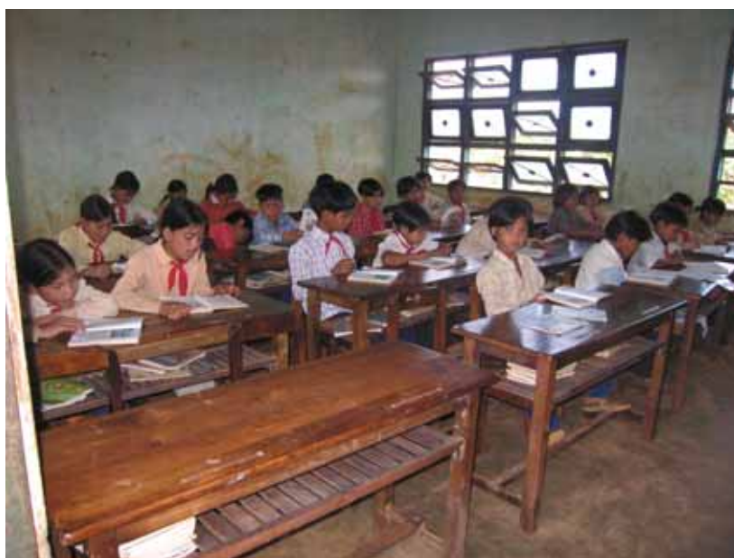
Classroom infrastructure is often worn or deficient as seen in this classroom's undecorated and stained walls. Photo taken at Lo Pang primary school, Mang Yang district, Gia Lai province
